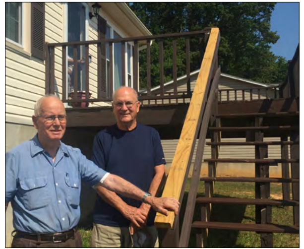
June Carpenters Project: Frank Cuthrell and Chuck Sampson repair a hand rail.
